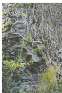
Deterioration at the corner of that wall.
