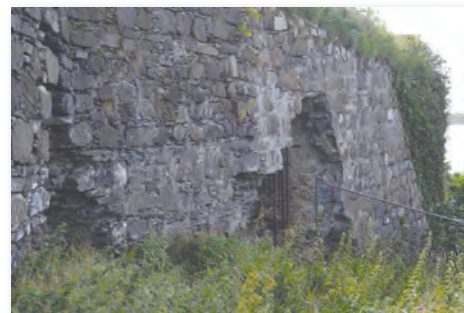
Deterioration at the base of another wall of the castle.
